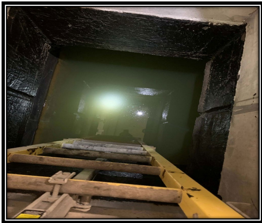
Figure 1 – Fire System Water Tank at Edith Green-Wendell Wyatt Federal Building 2
