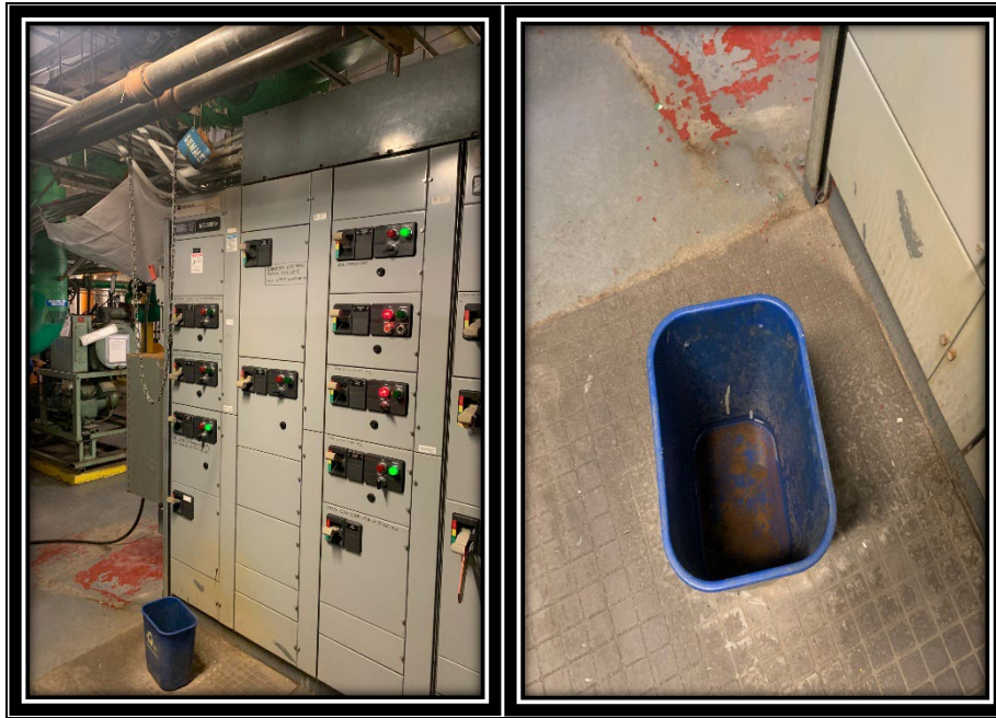
Figure 3 – Motor Control Center at Jacob K. Javits Federal Building with Blue Recycling Bin to Collect Water from Leaking Valve 6
