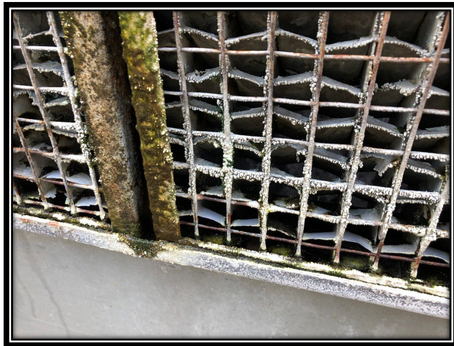
Figure 4 – Biological Growth and Scaling on the Cooling Tower at the Sam Nunn Atlanta Federal Center 9
